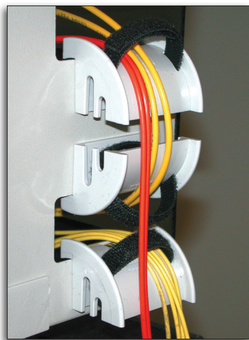
Patch Panel Egress
