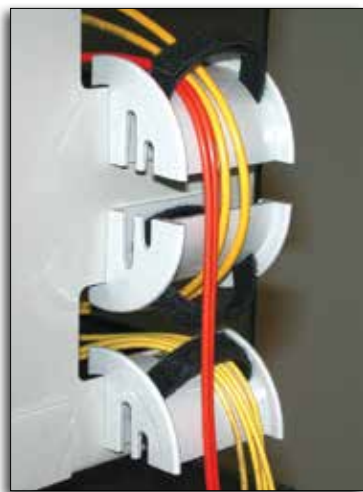
Patch Panel Egress
